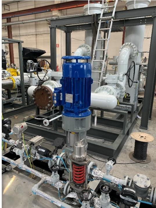
Ammonia Flow Control Unit
