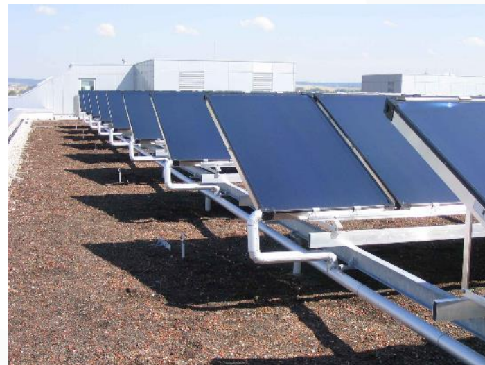
Source photo : Solahart (Solar Cooling Audi – Germany)
